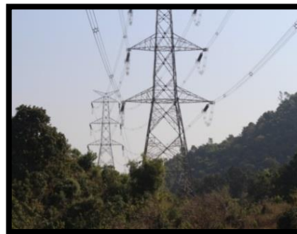
Power Grid Transmission Line
